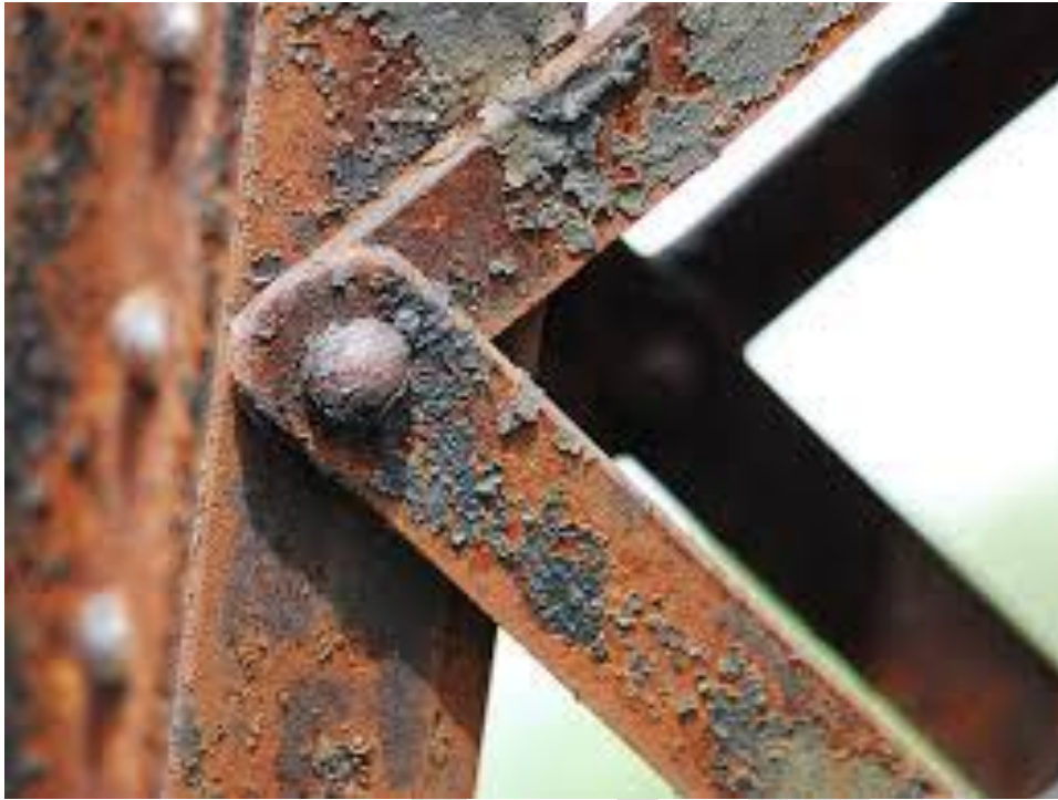
Fig.3: Corrosion of structures.
